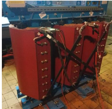
Figure 1 – Distribution transformer 10/0,4 kV under measurement
