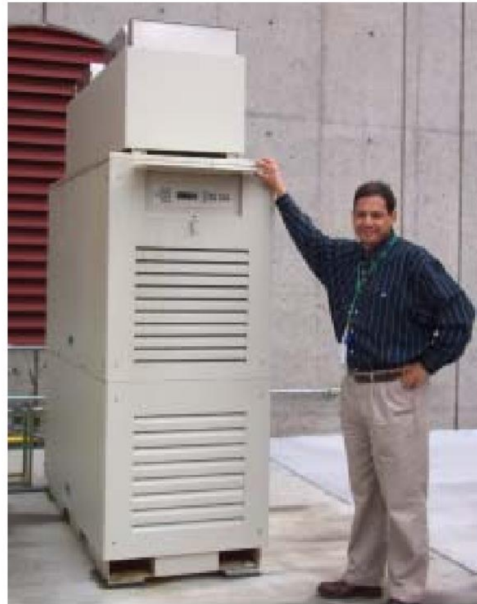
Capstone microturbine - 60 KW
